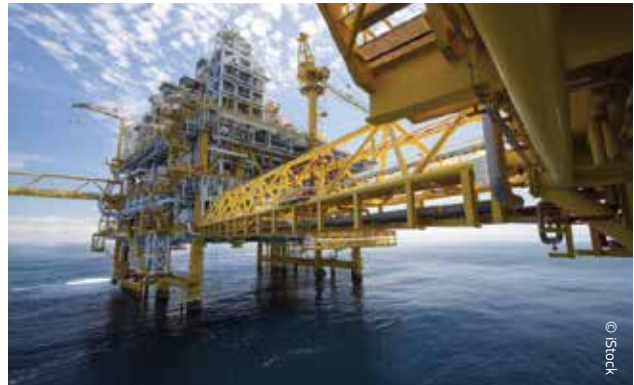
All oil and gas installations operating in EU waters are covered by laws ensuring that the highest safety standards are applied.
